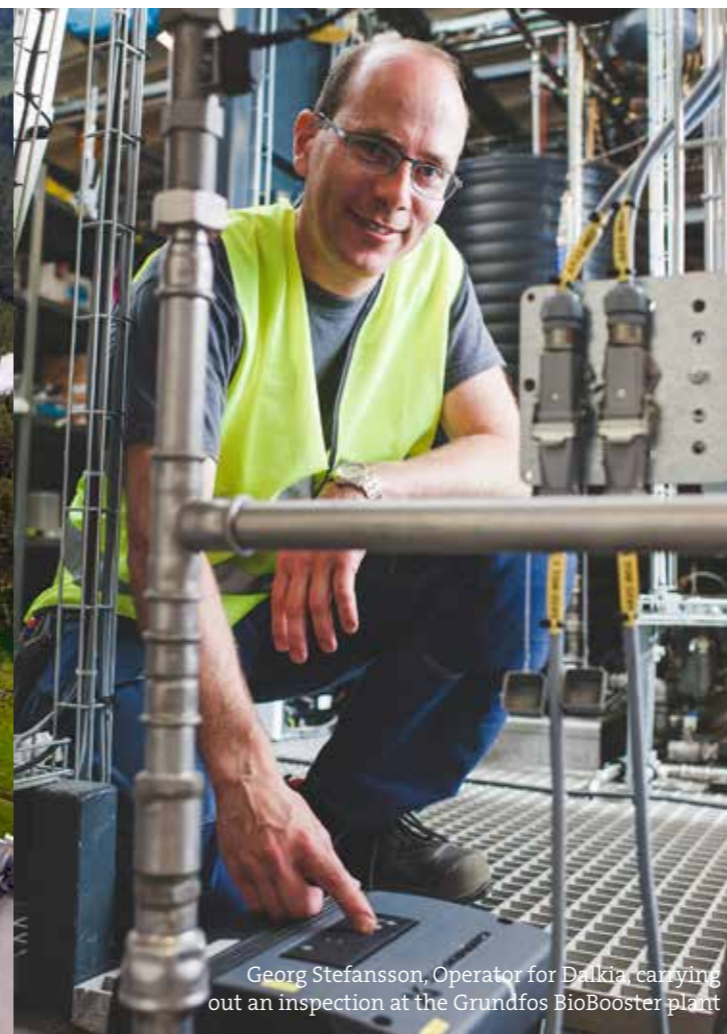
Grundfos BioBooster on-site at the Arla Foods milk processing plant, Vimmerby
